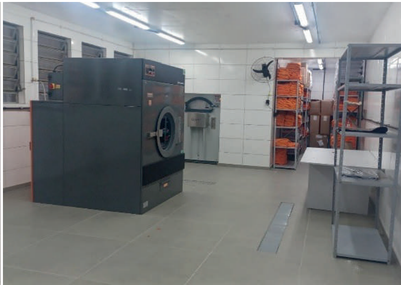
Laundry facility installed at PASC
